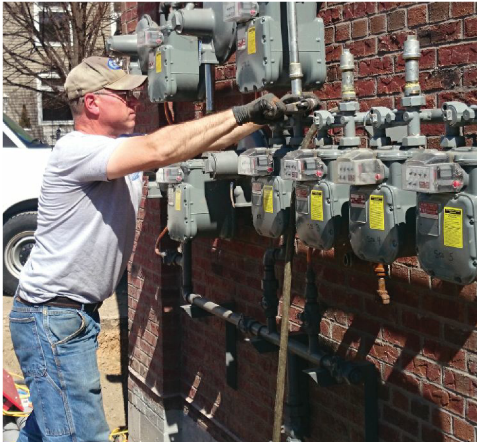
Many contractors, such as Jerry Grendahl, CEO, Grendahl Mechanical Inc., Edina, Minnesota, believe that, one day, on-demand service companies may be a threat to professional HVAC contractors.
